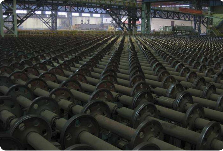
A large cooling bed for steel plates. Each wheel is supported by four high temperature bearings.
